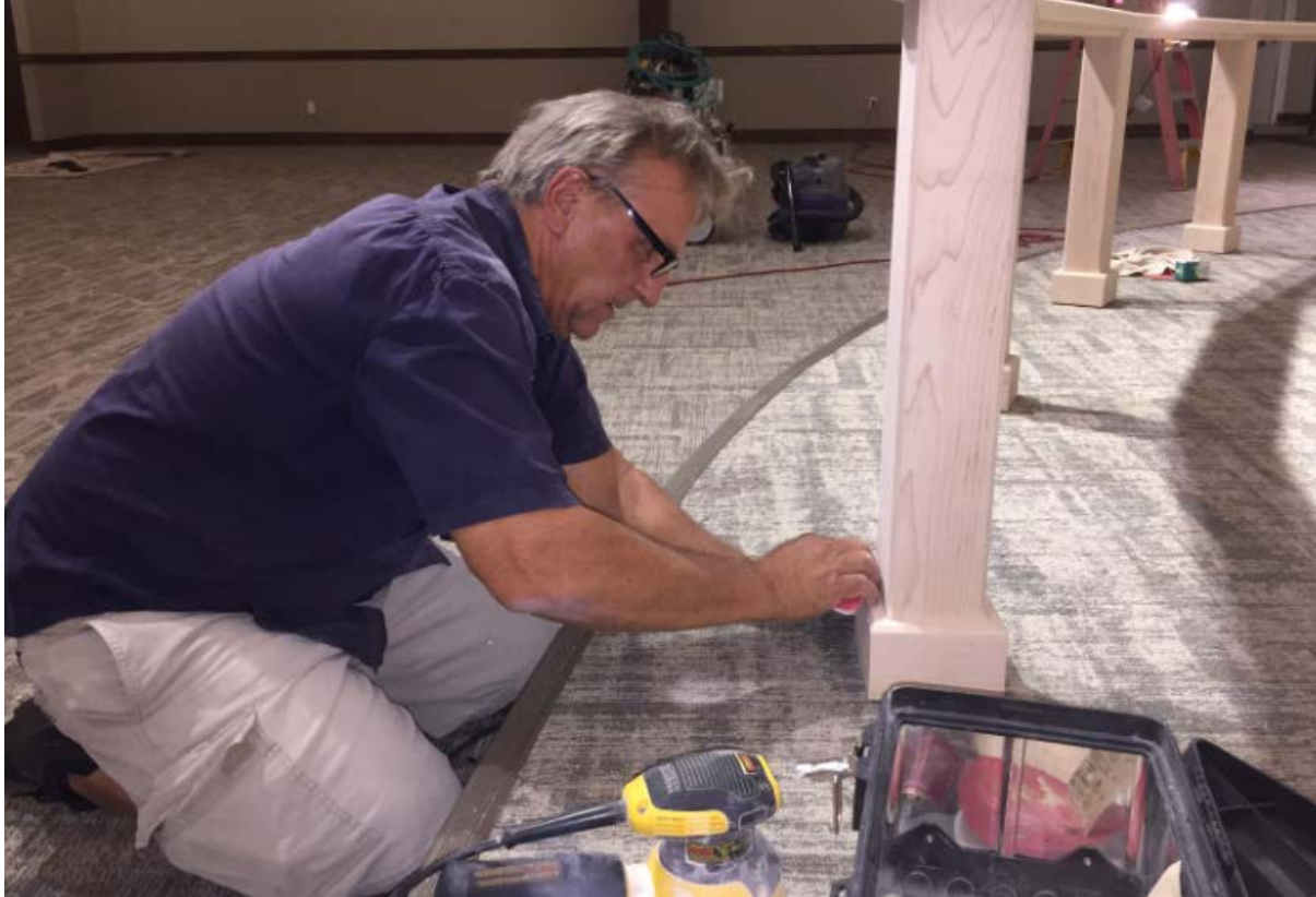
ABOVE: Larry Benton, with Larry the Cabinet Guy of Vero Beach, finishes the maple Altar Rail he constructed for the Worship Center in Christ Church Vero Beach. Located at the corner of State Road 60 and 6 th Ave. in Vero Beach, Church services are scheduled to begin in mid-June.
